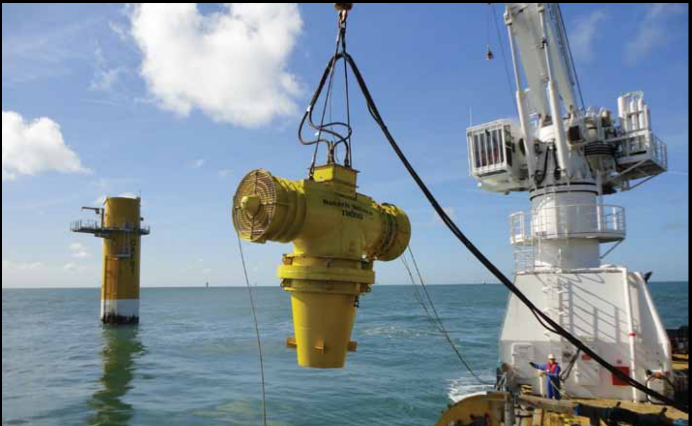
The T8000 being deployed from the Bourbon Enterprise to excavate cable transitions into monopile J tubes
